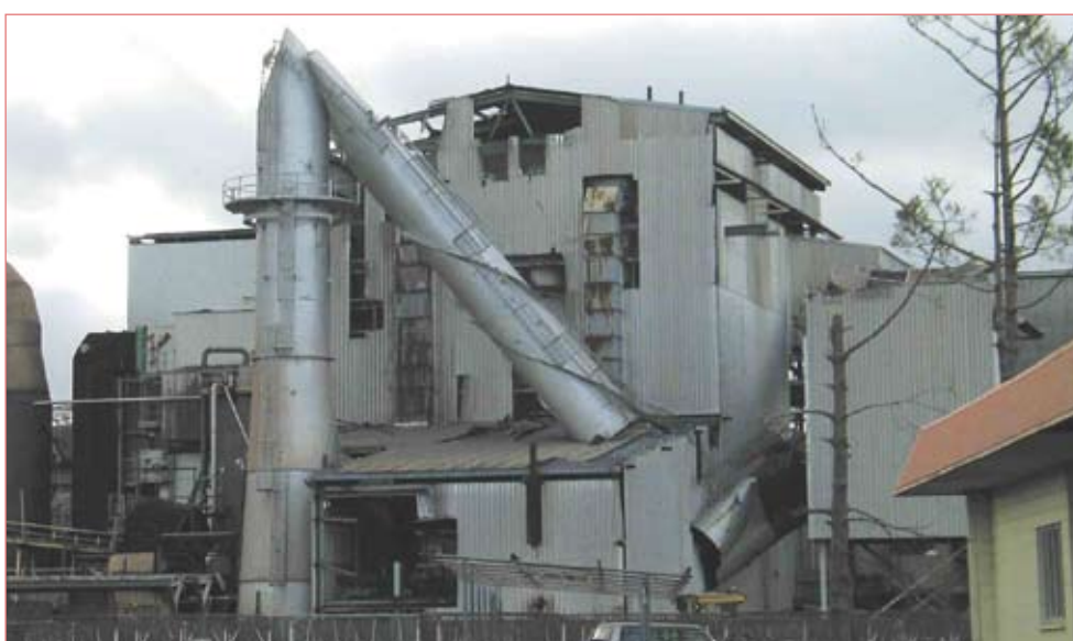
Cyclone damage to Mourilyan Mill.
